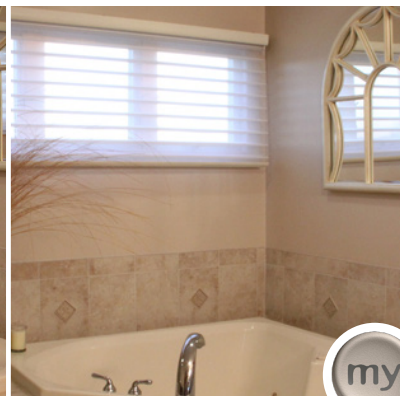
"MY" POSITION: The motorized sheer horizontal vanes are tilted open to diffuse light entering the room.
